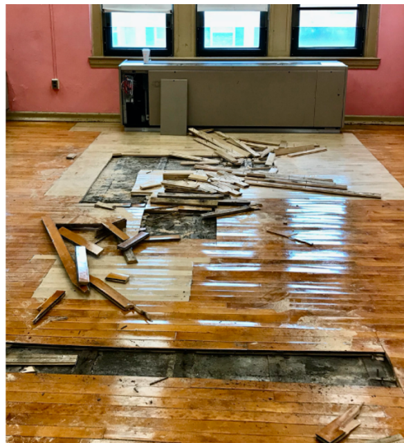
Photo 7 – Elem. Classroom — Repeat flooding from malfunctioning classroom unit ventilator resulting in extensive damage and mold growth to newly installed flooring — the original flooring was replaced for the same reason just a few weeks earlier. An example of what happens if the “root causes” are not addressed and also issues related to inadequate governance, oversight, and management
