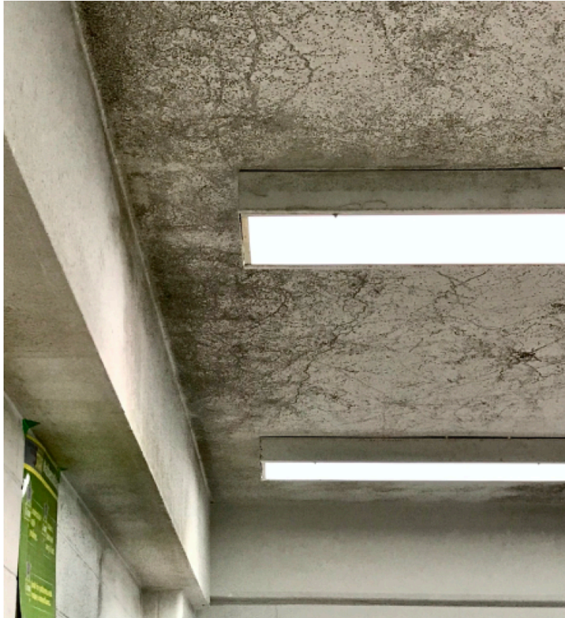
Photos 4 & 5 – Mold Growth on Ceiling and Wall of Occupied Elem. Classroom - according to teacher, condition present for months — Associated with HVAC System Problems
