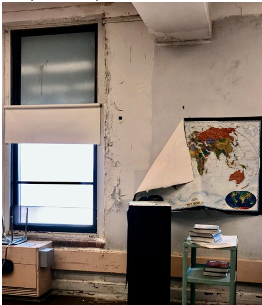
Photo 1– Elem. Classroom — Antiquated classroom unit ventilator, damaged/flaking lead paint, and obvious signs - and damage associated with - moisture and water intrusion.
