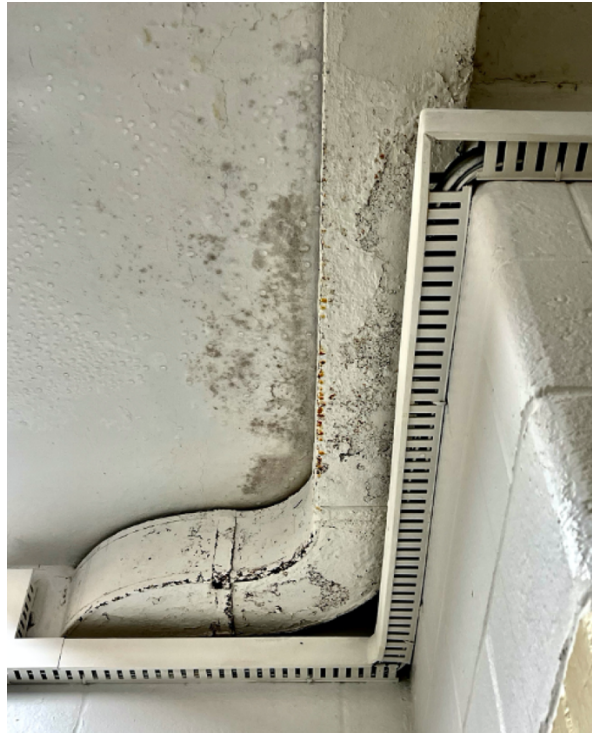
Photo 6 – Elem. Bathroom – Mold growing on ceiling and ductwork
