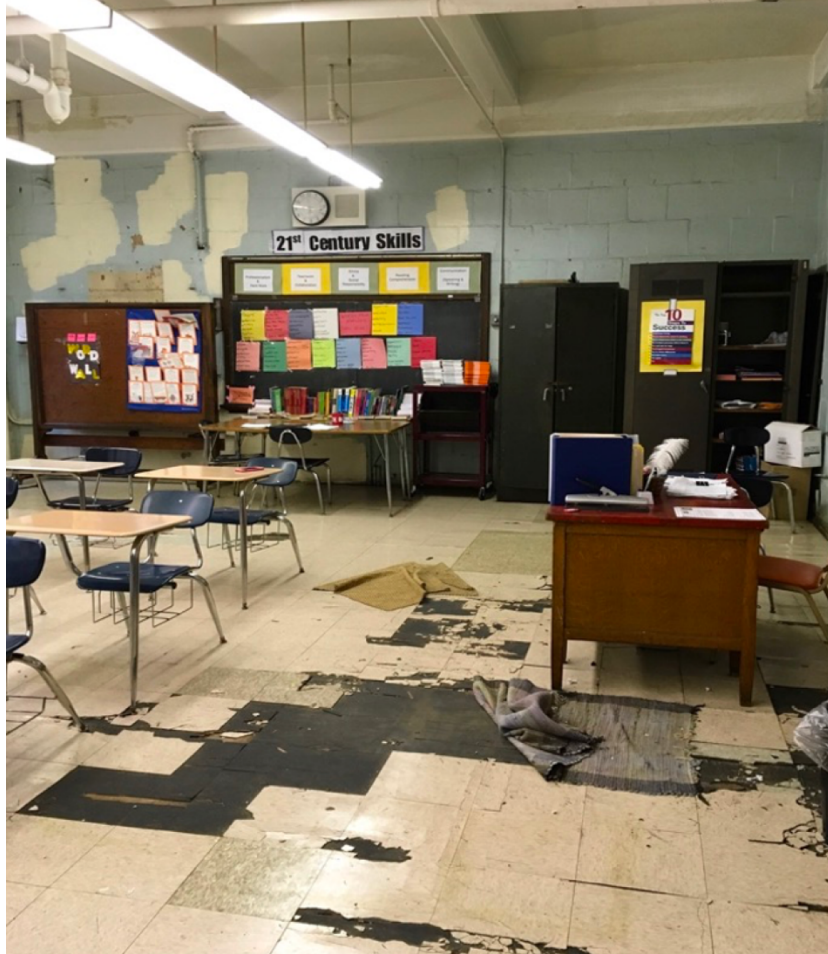
Photo 8—High School— Teacher described the conditions as existing for several months. The floor tile is an asbestos-containing material.
