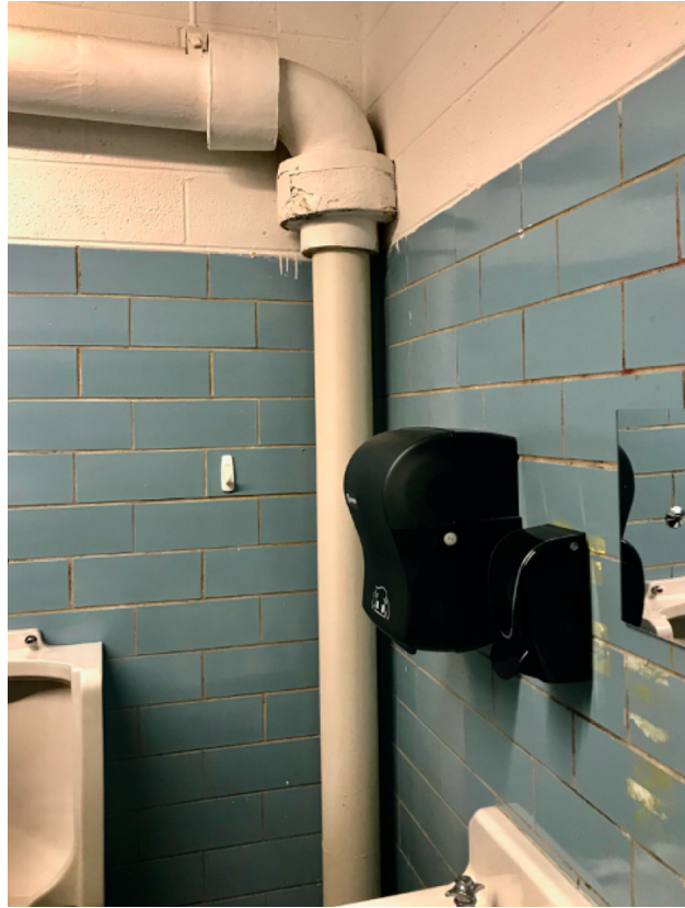
Photos 11 & 12- Bathroom — Accessible, damaged asbestos insulation between urinal and sink — this condition is present in multiple locations.
